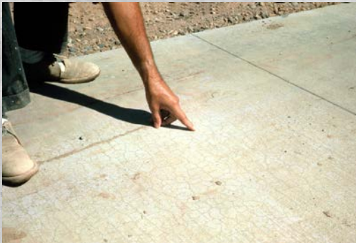
Crazing on exterior flatwork
