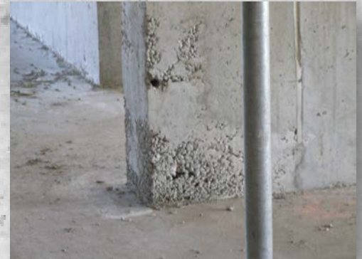
Honeycombing in a residential shear wall
