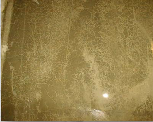
Crazing on a residential garage floor slab
