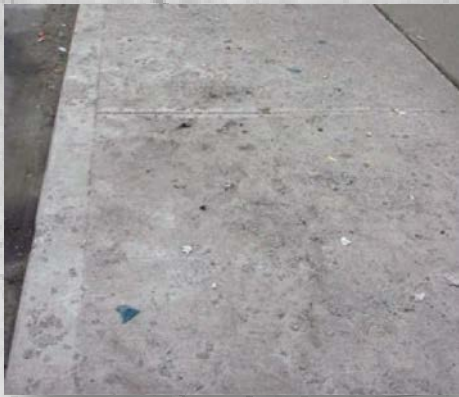
Light scaling of a concrete sidewalk
