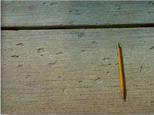
Mortar flaking on a concrete sidewalk – note that the aggregate is sound and only the mortar above the aggregate has failed
