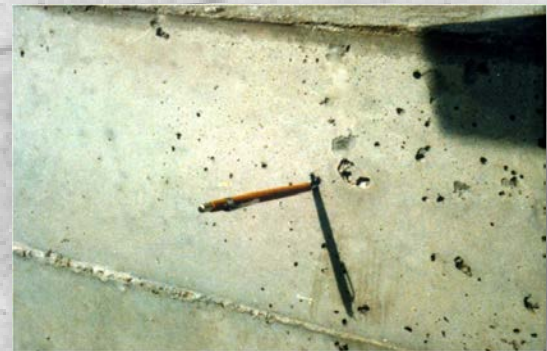
Bugholes on a plywood formed surface
