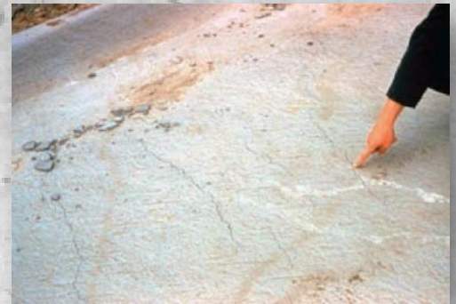
Plastic shrinkage cracks on exterior flatwork
