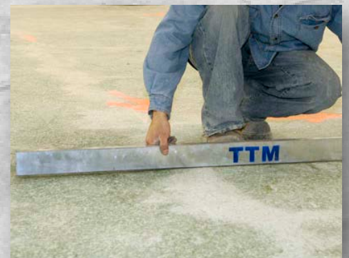
An example of a wavy concrete surface
