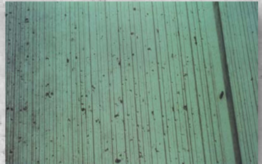
Bugholes on a concrete surface created with a form liner
