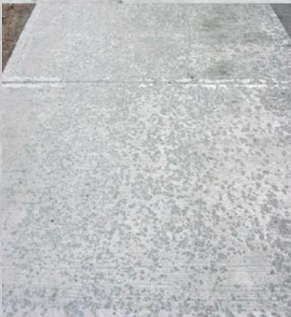
Medium scaling of a concrete sidewalk
