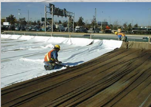
Proper concrete curing practices significantly reduce instances of concrete scaling
