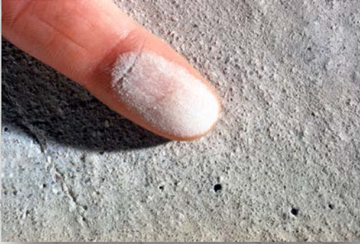
An example of a dusting concrete surface
