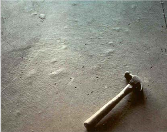
Blistering concrete surface
