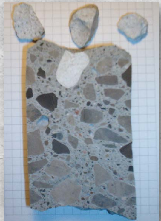
A cross-sectional view of a concrete core taken from a popout area – note the large chert particle in this limestone aggregate source that is responsible for the popout
