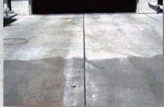
Discolouring of a residential driveway due to the use of calcium chloride (accelerator) in only one of the two loads
